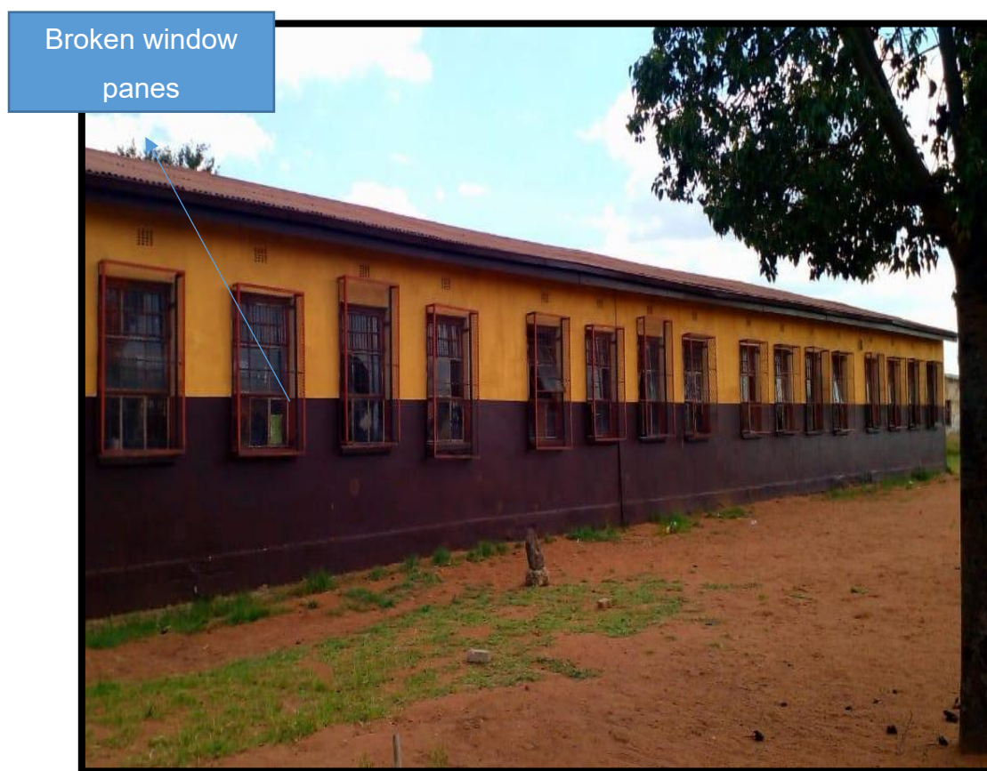
Figure 3.2: Participating school: indication of broken windows as some of the difficult conditions in Rekopantswe Circuit
