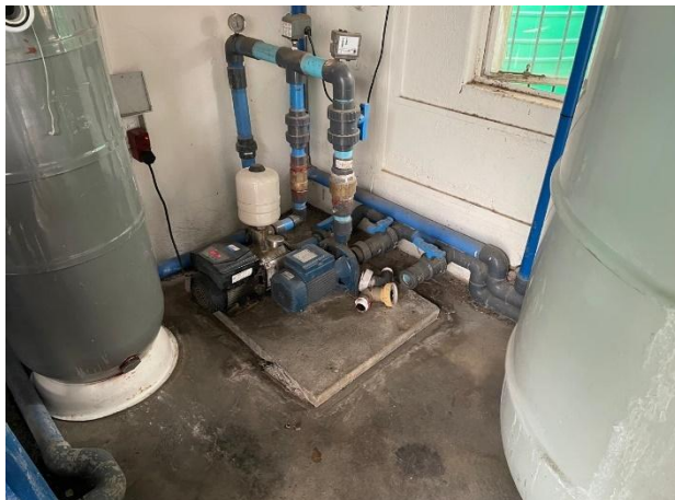
Figure 4.4 Water abstraction and pump system at Ngala Safari Lodge
