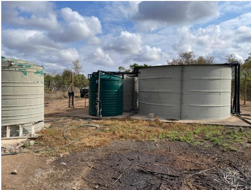
Figure 4.14 Enclosed wastewater treatment plant
