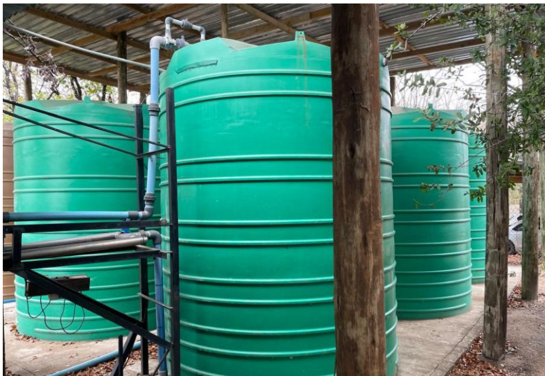
Figure 4.5 On-site water storage tanks used for lodge water supply
