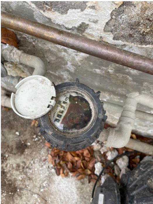
Figure 4.6 An on-site water meter is used to monitor lodge water consumption
