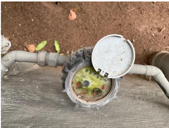
Figure 4.13 On-site Ngala Tented Camp water meter example 2
