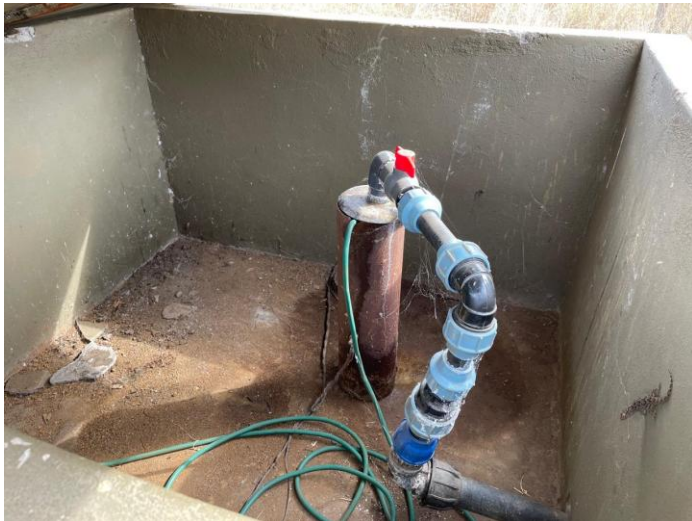
Figure 4.9 Enclosed borehole abstraction point at Ngala Tented Camp
