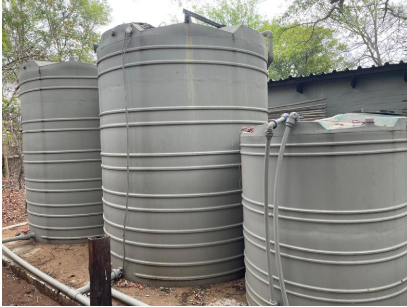
Figure 4.11 Ngala Tented Camp water storage facility
