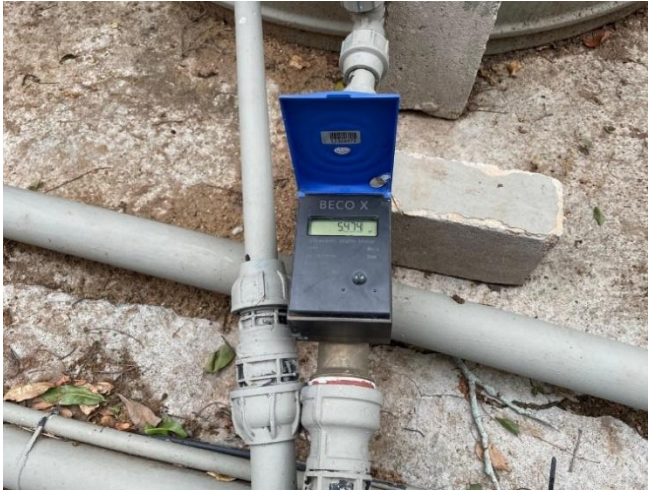
Figure 4.12 On-site Ngala Tented Camp water meter example 1
