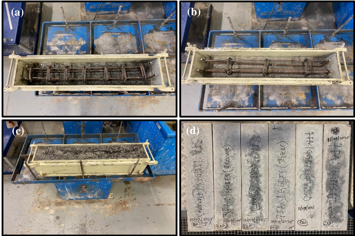
Fig. B7: Beam casting stages (a) placement of flexural rebar in the mould (b) placement of shear rebar in the mould (c) freshly cast GPC beam (d) hardened beam after demoulding
