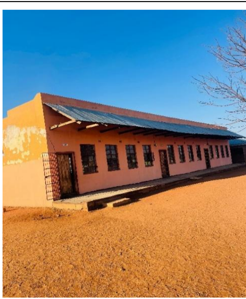
Image 2: Old damaged buildings
