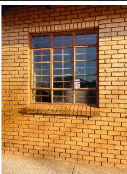
Image 4: Classrooms with broken windows
