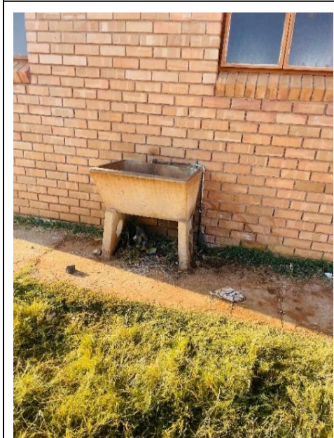
Image 7: Poor sanitation (non-functional water basin)
