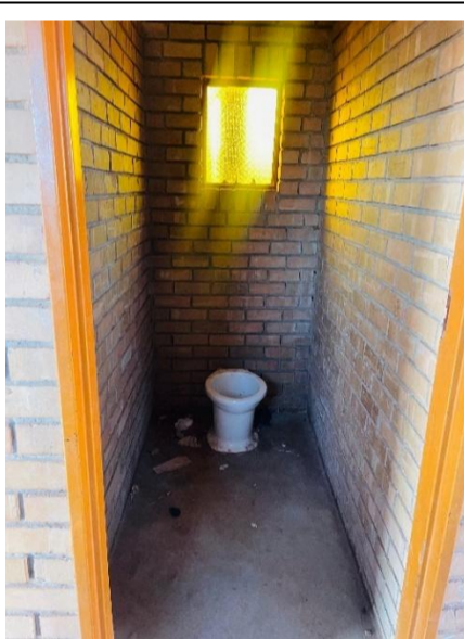
Image 6: Toilets with no doors
