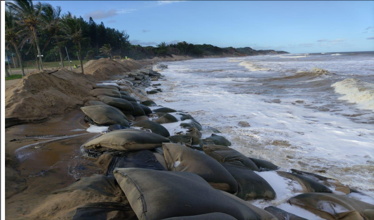
C: 2024/2025 - Severe storm surges resulting in the shifting of geotextile sand bags causing sand to erode under the bags. Sand replenishment used as a soft engineering approach (Source: Alakram, 2025).
