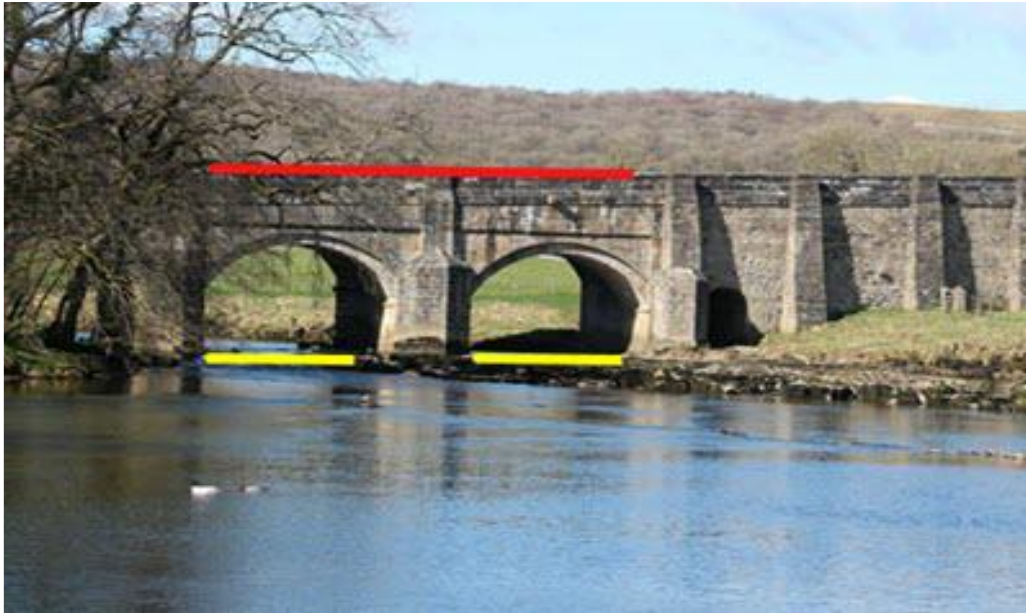
Figure 3.17: The elevation of the bridge (in red) is higher than the elevation of the water passing under the bridge (in yellow) (Adapted from Bastrom & Kirby, 2021).
